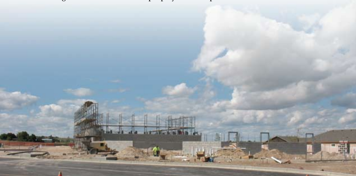
Construction underway on the Lakeview Bible Church building in a growing area of Nampa, Idaho. Lakeview is one of three recent additions to the FEC family.
